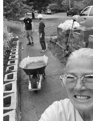
Tone, Doris, Shannon building the retaining wall in front of Bread and Roses
