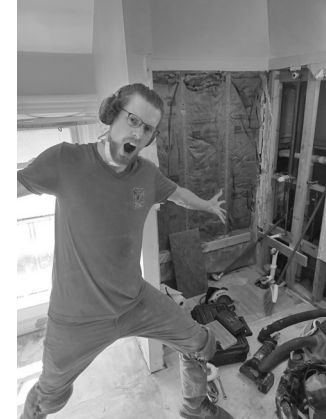
Hannah House bathroom got a new tub, floor tile, and rotten underlayment was replaced!
